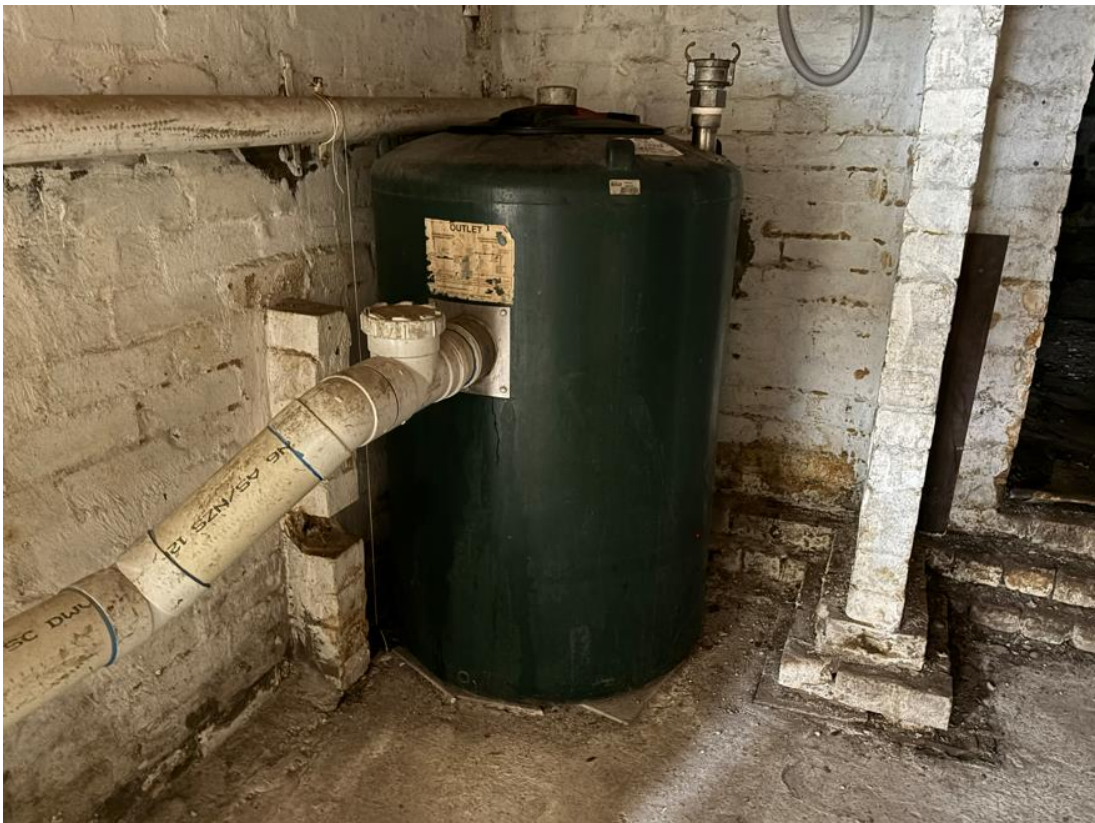
Photograph 4 View of above ground grease trap (28 Pacific Highway).
