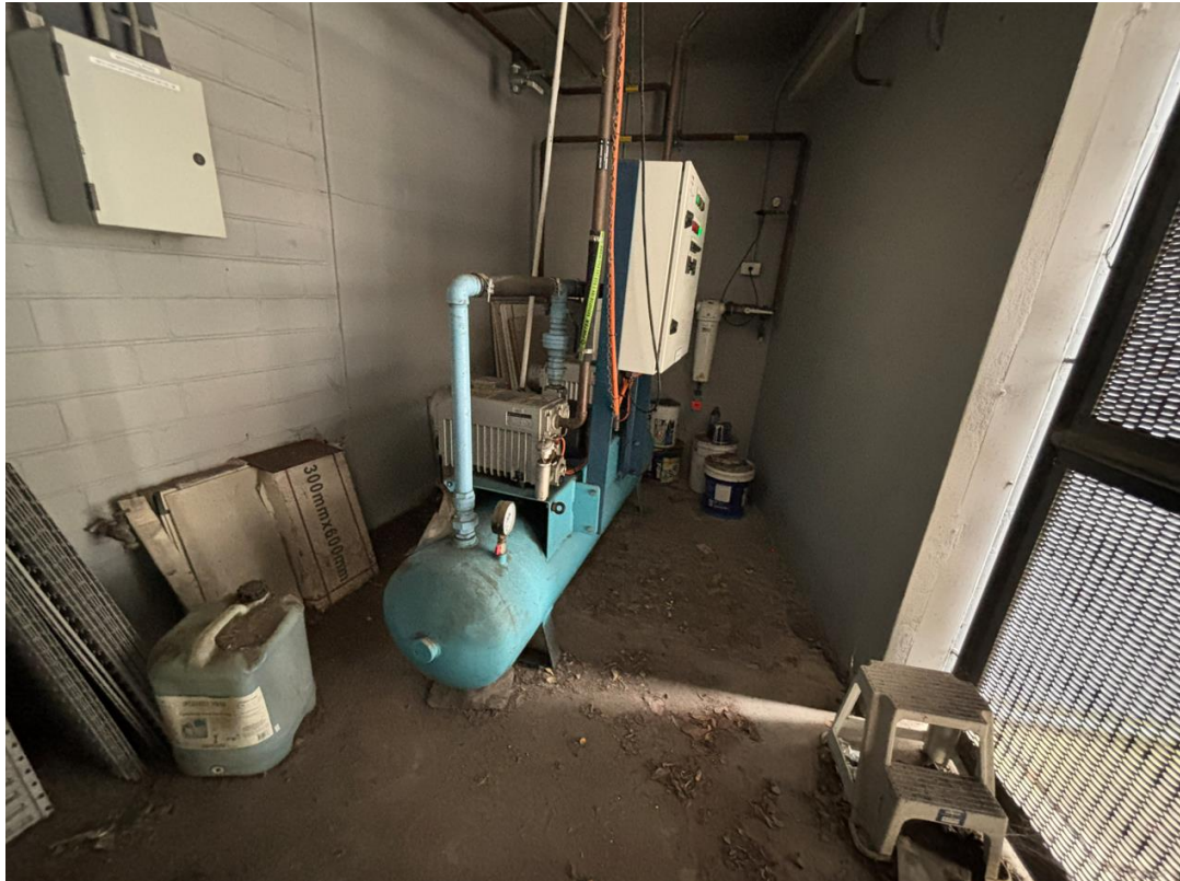
Photograph 15 View of oxygen gas supply room within basement (34-38 Pacific Highway).
